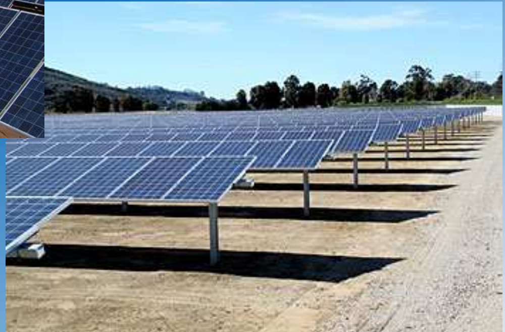
1,1 MW - Ventura County Waterworks District, Moorpark, CA , 2013
