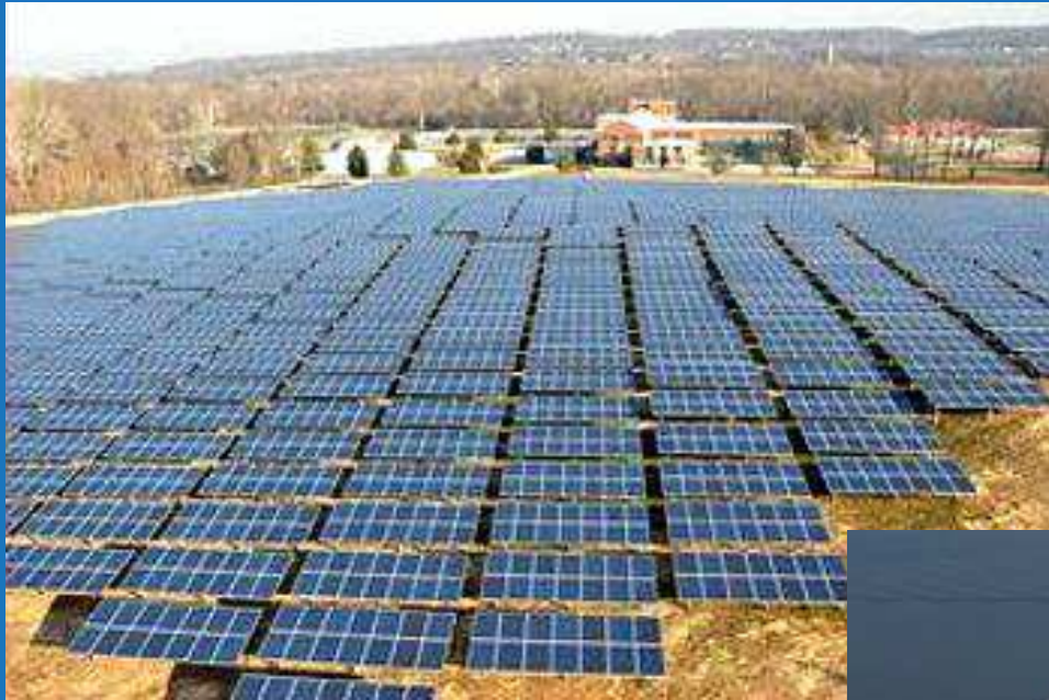
1,8 MW - Aqua Pickering Solar Farm at the Pickering Wastewater Treatment Plant, Chester County, Pennsylvania, 2012
