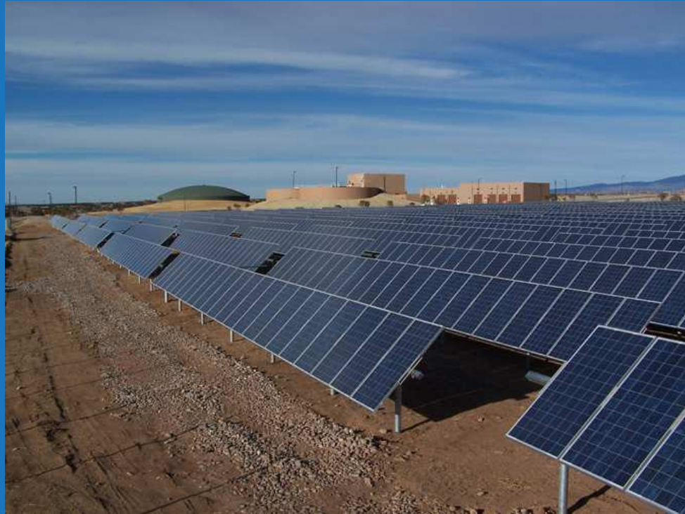
1 MW - City of Santa Fe and Santa Fe County, Buckman Direct Diversion, Nowy Meksyk, 2011
