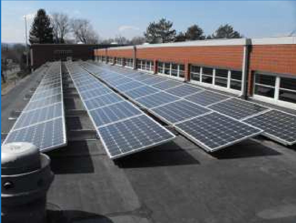
50 kW – Water & Sewer Department, City of Binghamton (New York), 2011
